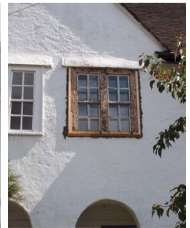
Timber windows can be easily repaired, prolonging the life of the window and keeping the character of the house.
