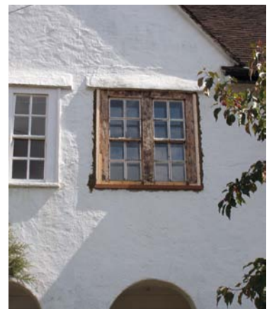
Timber windows can be easily repaired, prolonging the life of the window and keeping the character of the house.
