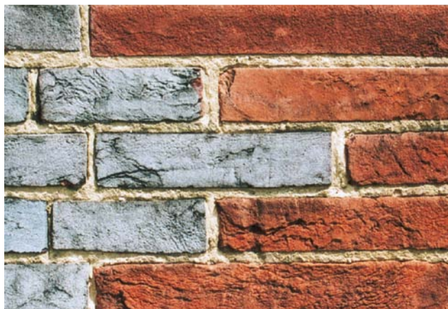
(Unpointed wall) Soft mortar encourages drying out, enhances the beauty of the bricks and makes them less liable to damage when a wet wall freezes
