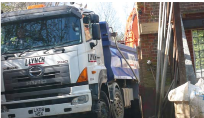
There was much consternation on the HGS list when 13 Hampstead Way almost disappeared overnight. The owner of the house, which overlooks the Heath, had been given permission for a certain amount of demolition preparatory to installing a basement which would have resulted in there being very little evident change to a rather handsome house. The Trust, on the case the next day, found that contractors had been overenthusiastic in demolishing all but the front and side walls and a chimney stack. Barnet and the Trust have taken action to ensure that the owners, at considerable cost, restore the house to exactly the same specifications as before. Meanwhile the pictures here show the effect a basement excavation has on the street and surrounding neighbours.
