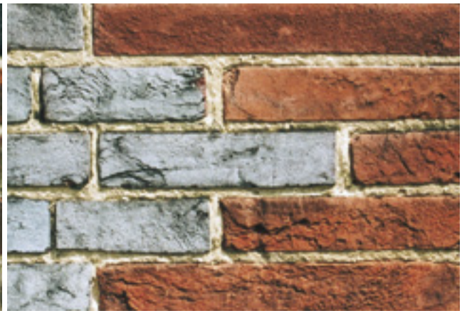
(Unpointed wall) Soft mortar encourages drying out, enhances the beauty of the bricks and makes them less liable to damage when a wet wall freezes
