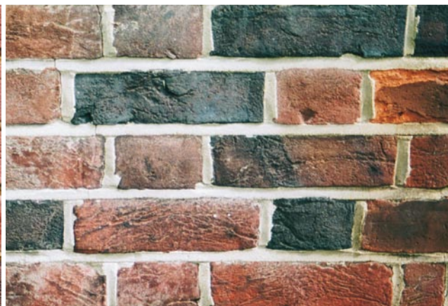
(Badly pointed wall) Modern cement is stronger and rigid, cannot be removed without damaging the bricks and causes frost damage
