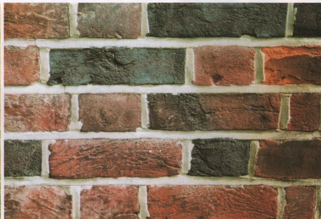
(Badly pointed wall) Modern cement is stronger and rigid, cannot be removed without damaging the bricks and causes frost damage.
