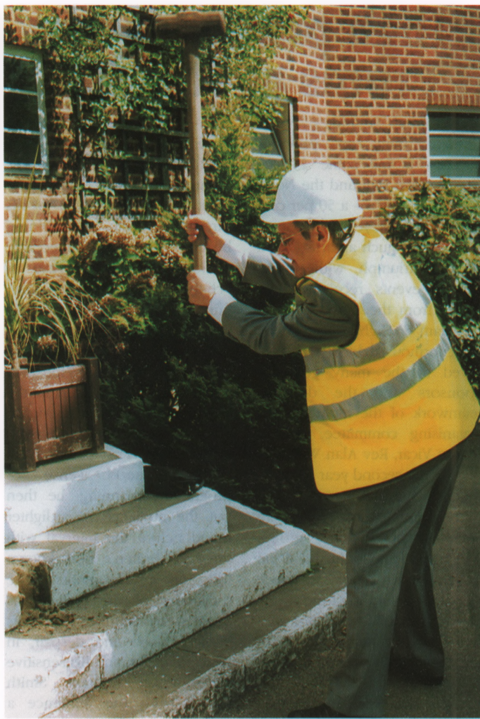
Rabbi Charles Emanuel strikes a ceremonial blow marking the opening stage of the rebuilding programme of the synagogue at Alyth Gardens
