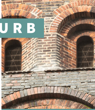
Missing tiles and poor pointing
