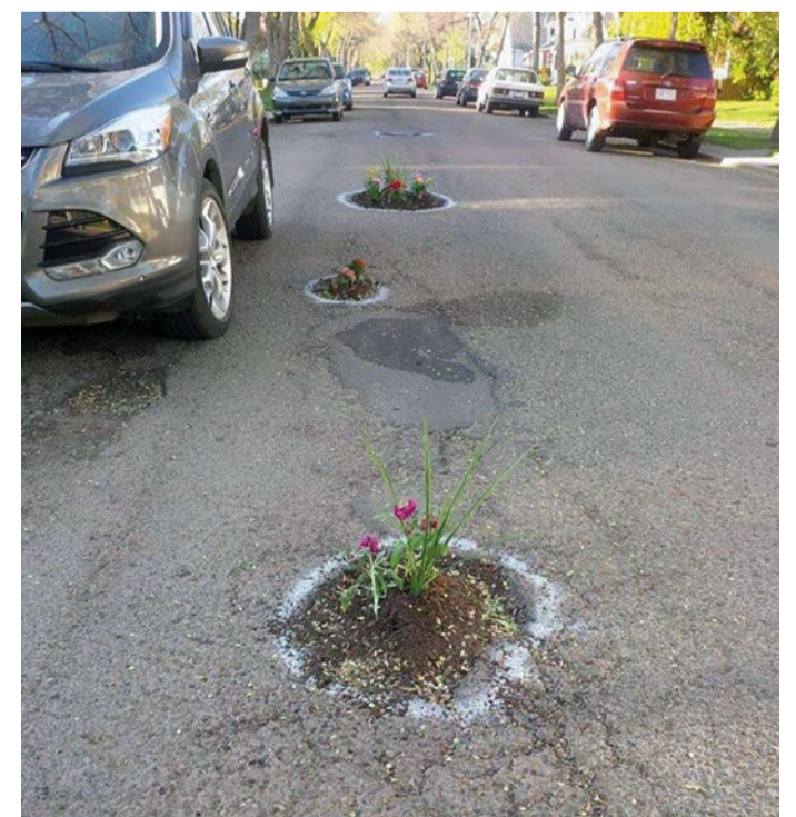
Pothole gardening; this photo of a rather original approach to filling potholes was posted on the RA's Facebook page. Will it spread, we wonder?
